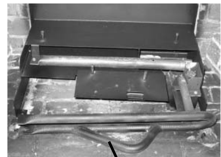
Front Burner Removed
